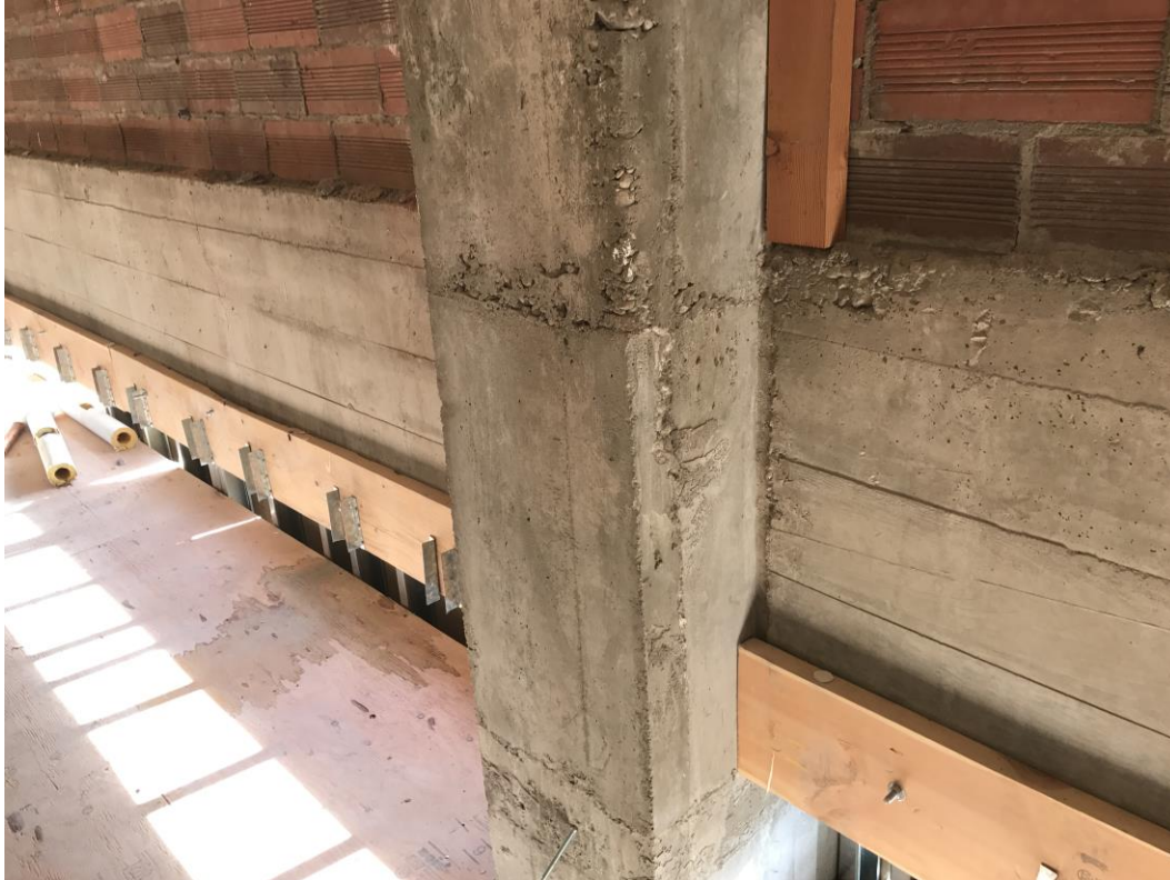
Cold joints in concrete columns (photo taken inside mechanical attic under mezzanine seating)
