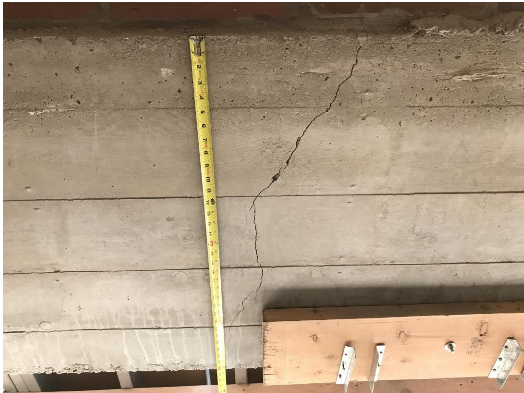
View of cracked bond beam (photo taken inside mechanical attic under mezzanine seating)
